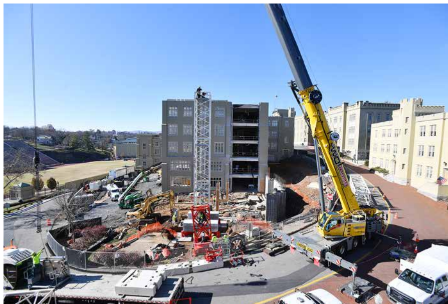
Crews install a 135-foot-tall crane during Thanksgiving Furlough for the Scott Shipp Hall renovation project.—VMI File Photo by Kelly Nye.
