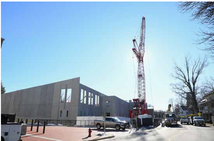
A crane towers over the Aquatic Center construction site on Main Street.—VMI Photo by H. Lockwood McLaughlin.
