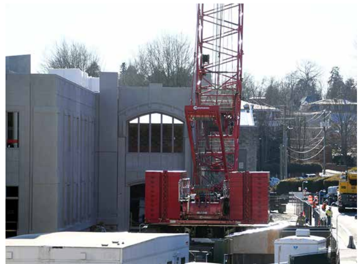
The entrance area of the Aquatic Center on Main Street takes shape during construction.—VMI Photo by H. Lockwood McLaughlin.
