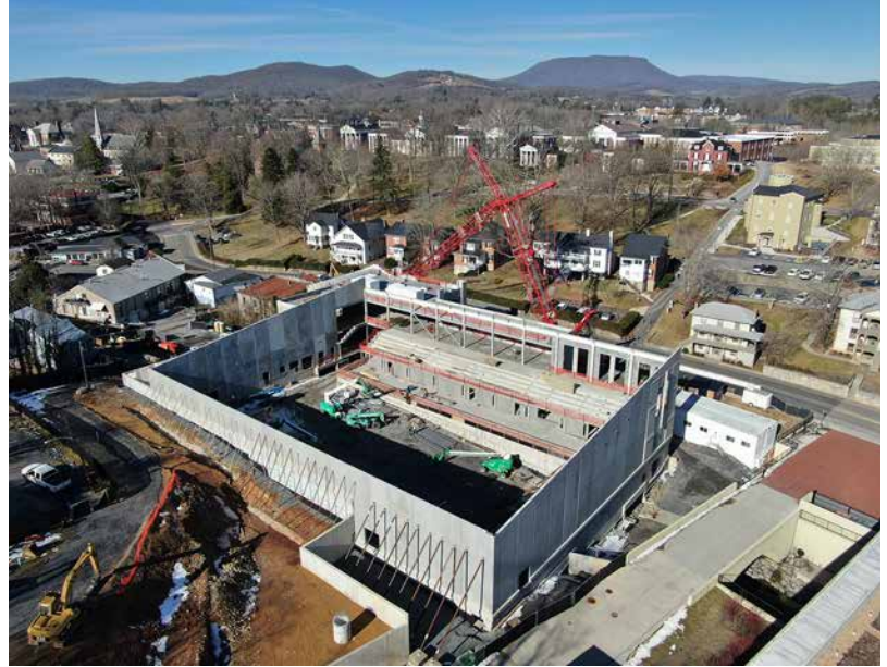
An aerial view of the Aquatic Center construction site shows the interior.—VMI Photo by H. Lockwood McLaughlin.
