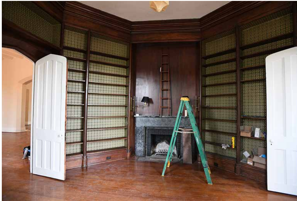
The library in the Superintendent's Quarters gets final touches in mid-June before furniture is placed.—VMI Photo by Kelly Nye.
