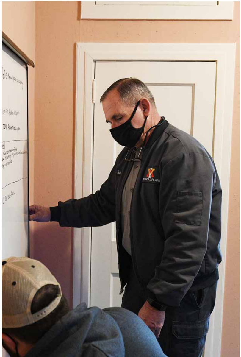
John Camper helps hang a white board in a recently repainted Human Resources office, one of the many buildings on post he oversees.—VMI Photo by Kelly Nye.
