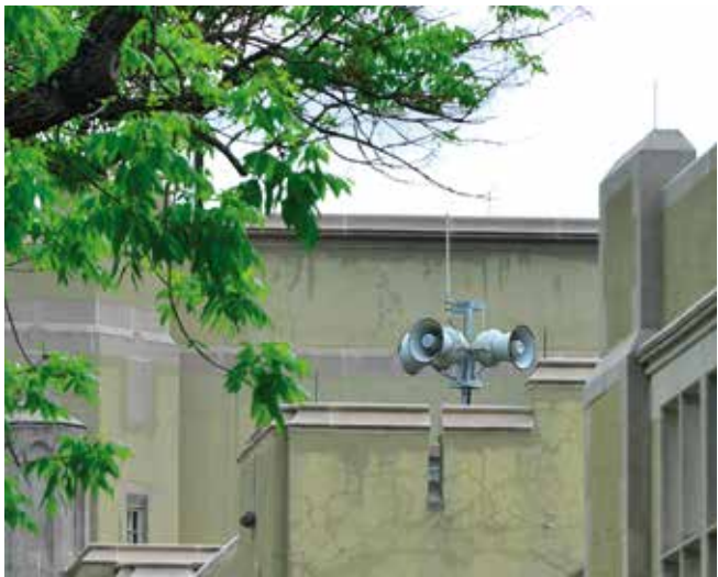
Loudspeakers atop Preston Library and other buildings are part of VMI's emergency notification system. In an emergency, the whole VMI community is notified immediately via loudspeaker, email, text, and voice-over-IP phone alert. An alert is also posted to the VMI website. – VMI Photo by Kelly Nye.
