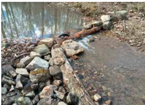
This newly constructed spillway is an ideal location for brook trout to spawn. The oxygenated water keeps silt from building up. – Photo courtesy of Michael Smith.
